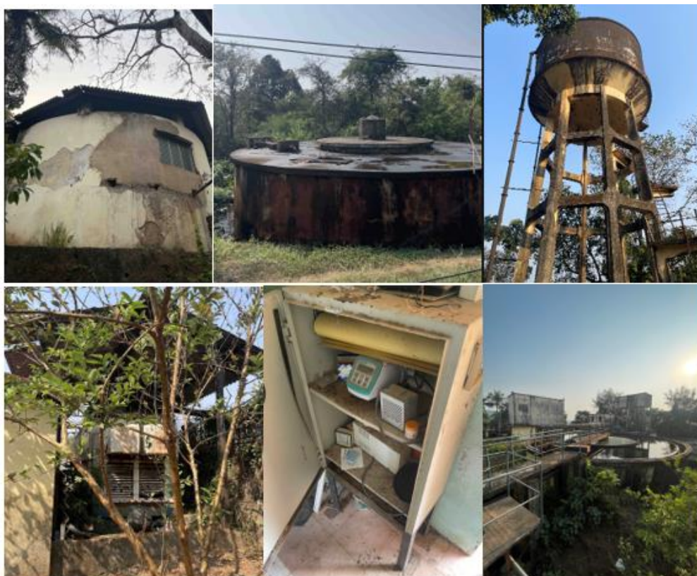
Photos of ageing water infrastructure at Canacona
