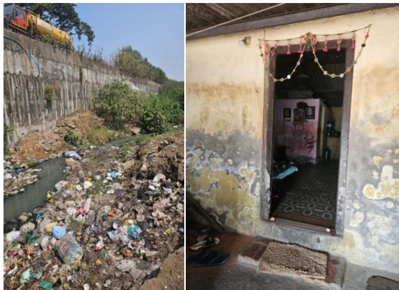
Photo 2 : Storm Water Drainage Situation and Flood Affected Household in Valsad
