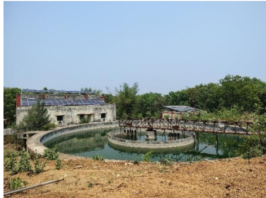
Figure 13: Clari-flocculator at WTP
