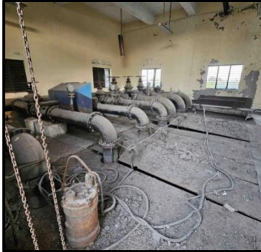
Photo 4 : Condition of Pumping Stations Post 2024 Floods
