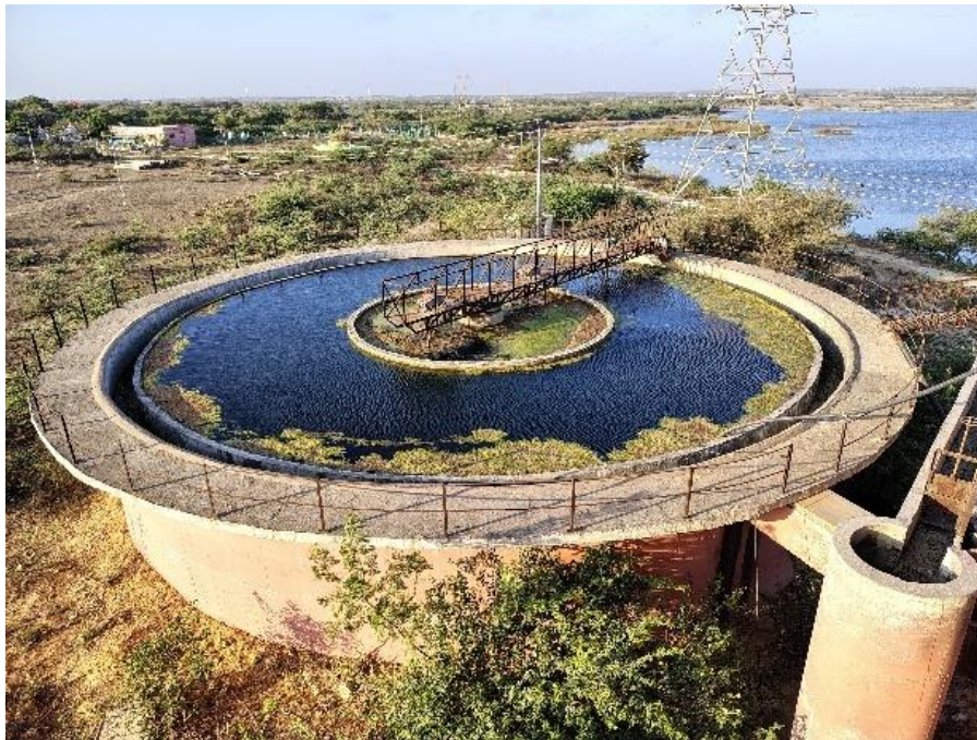
Figure 13: Non-functional clari-flocculator at WTP
