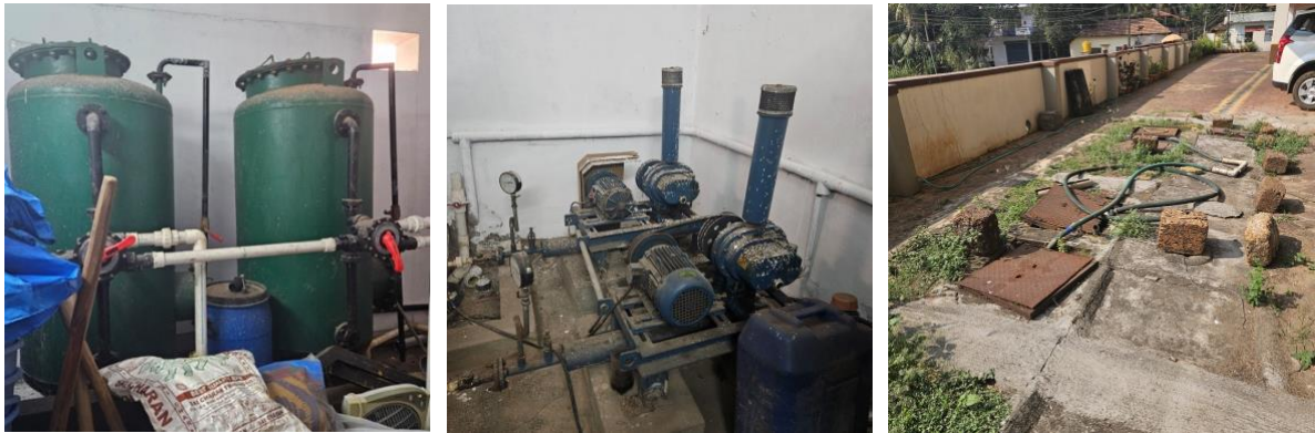
Photo : Decentralised Sewage Treatment Unit in Apartment Complex; Source: IITB Team
